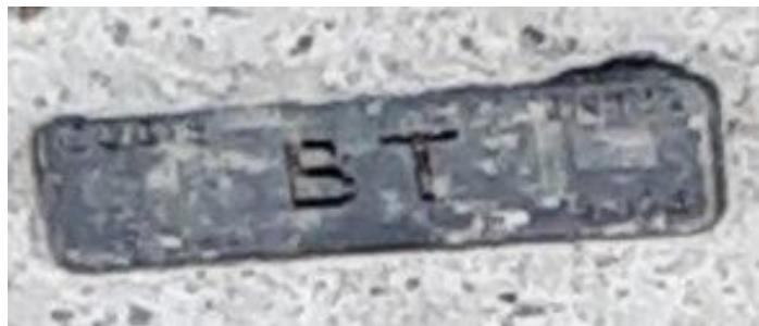
Current footway chamber id
